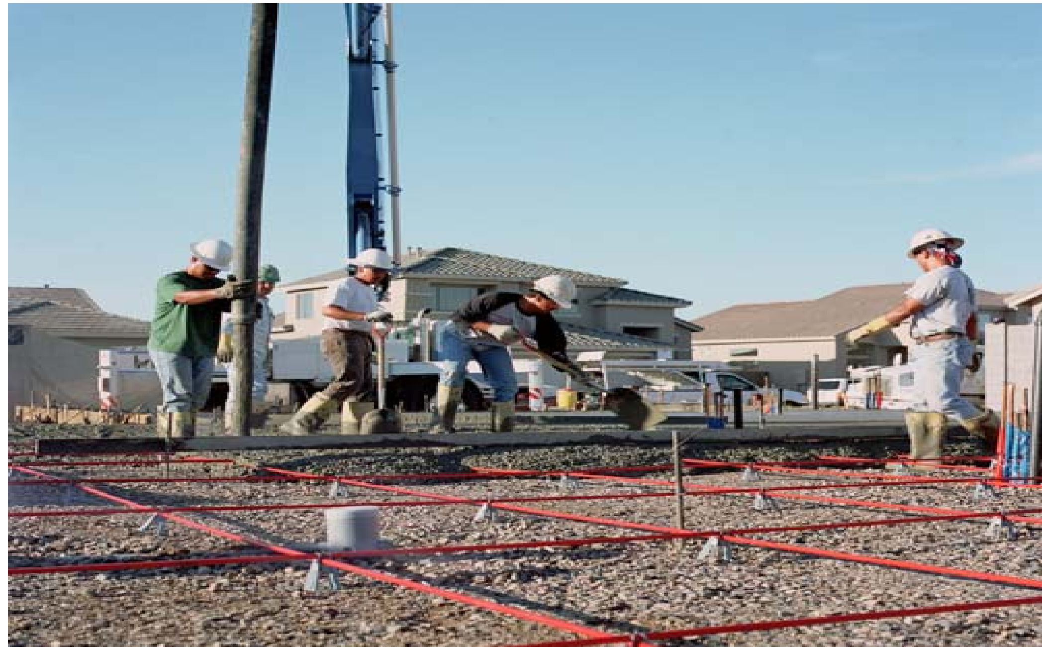
Good long term growth record and prospects Concrete placement for a Suncoast post-tension foundation slab in Arizona. Revenues from outside Suncoast's traditional Texan market are now three times the level in 2002, the first full year under Keller ownership, with good opportunities for further growth.
