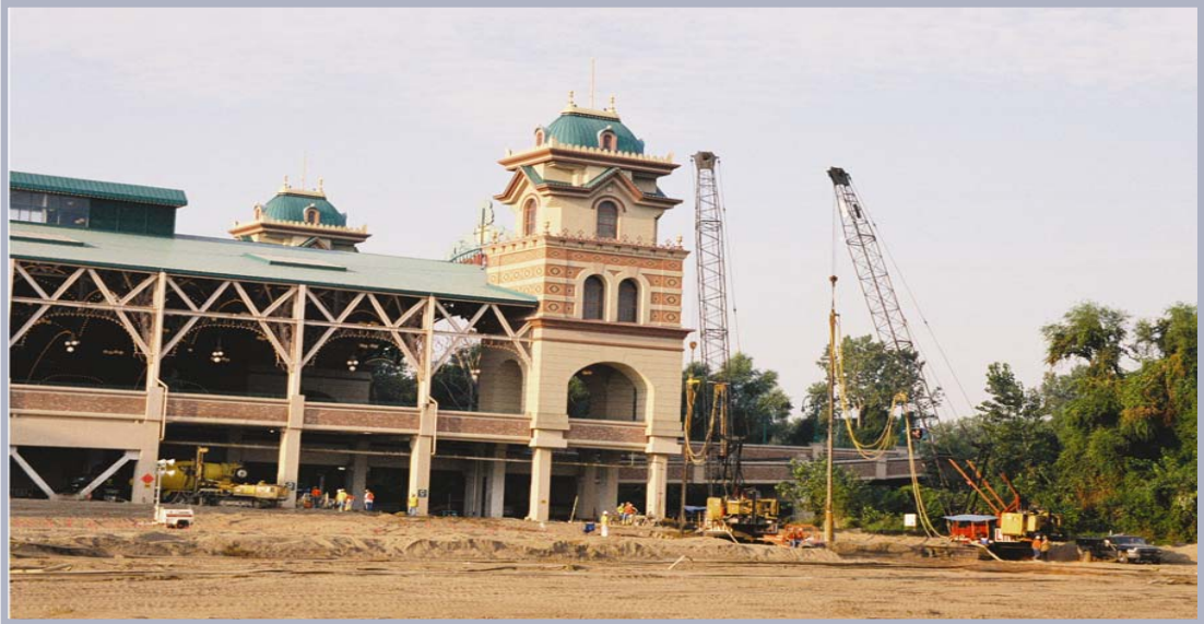
Hayward Baker Vibrocompaction, grouting, minipiles Casino, hotel and parking deck St Charles, Missouri
