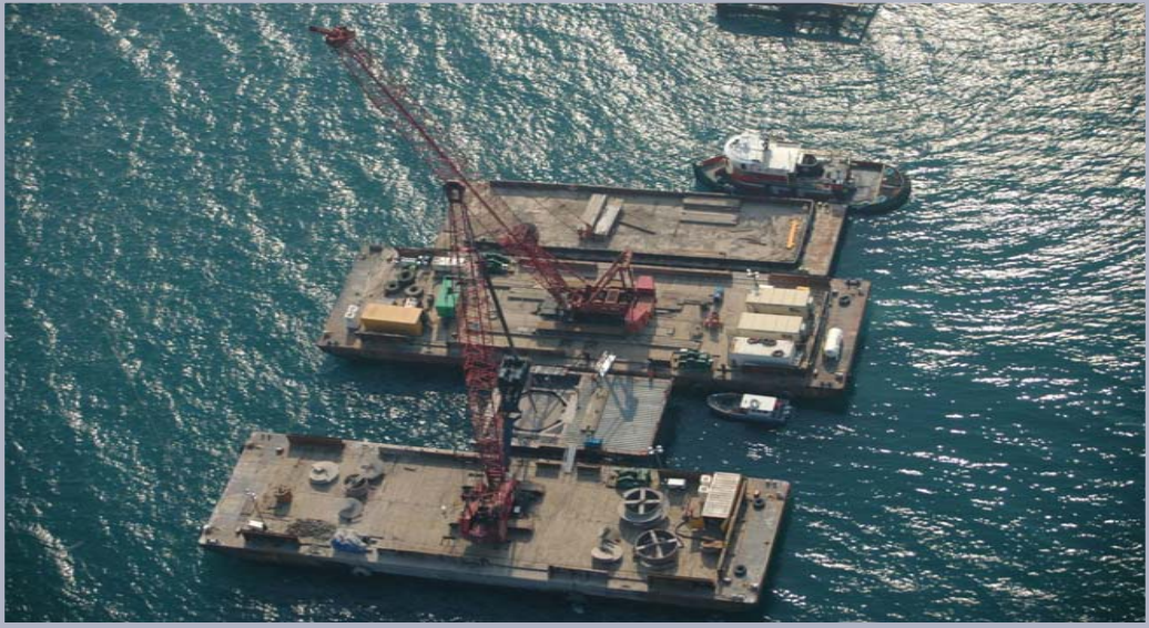
Case Foundation Large shafts Water intake shafts for new power station Lake Michigan, Wisconsin
