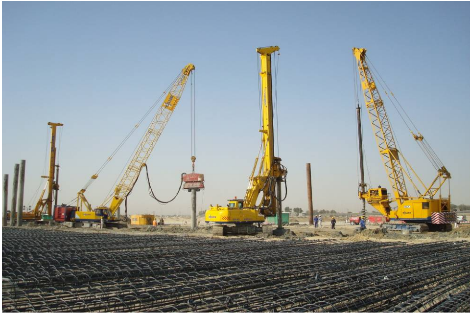
Foundations for petrochemical complex, Al-Jubail, SA Three contracts totalling c. €60m (£40m) Piling underway with peak activity by September
