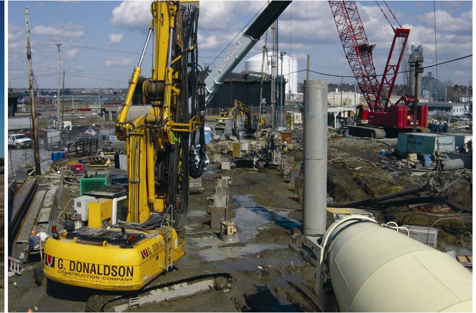
Hayward Baker (including Donaldson division) Combined Sewer Overflow System, Providence, RI Piling, excavation support and jet grouting Illustrates synergies from Donaldson acquisition
