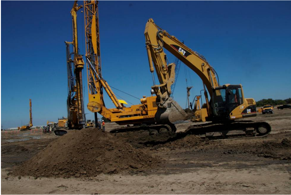
Hayward Baker & Anderson Pacific Ethanol Plant, Stockton, CA Vibro replacement and deep soil mixing Multi-company, multi-product site
