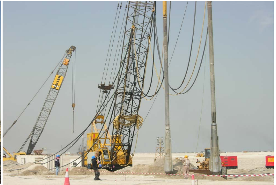
Sand compaction at Palm Deira ("Palm III"), Dubai Use of new S700 vibrators
