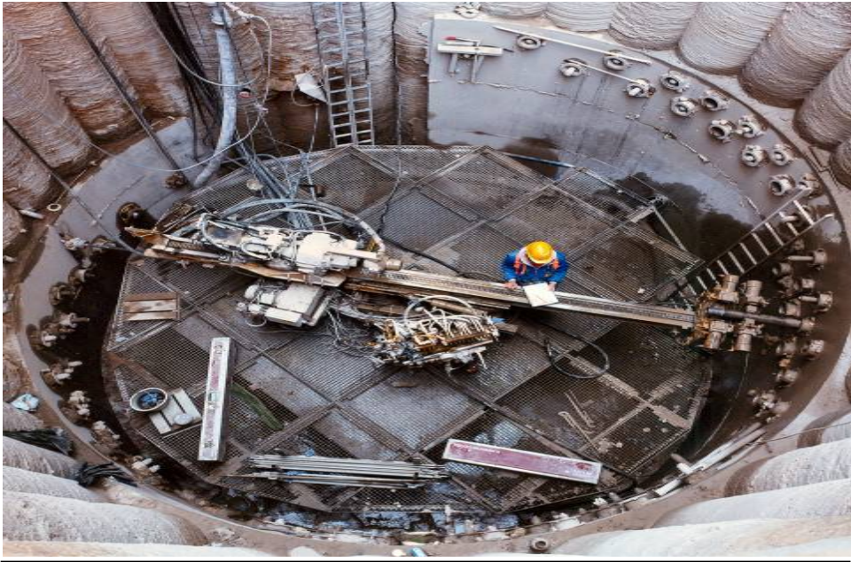
New railway tunnel in Leipzig Connecting North & South stations Compensation and cement grouting
