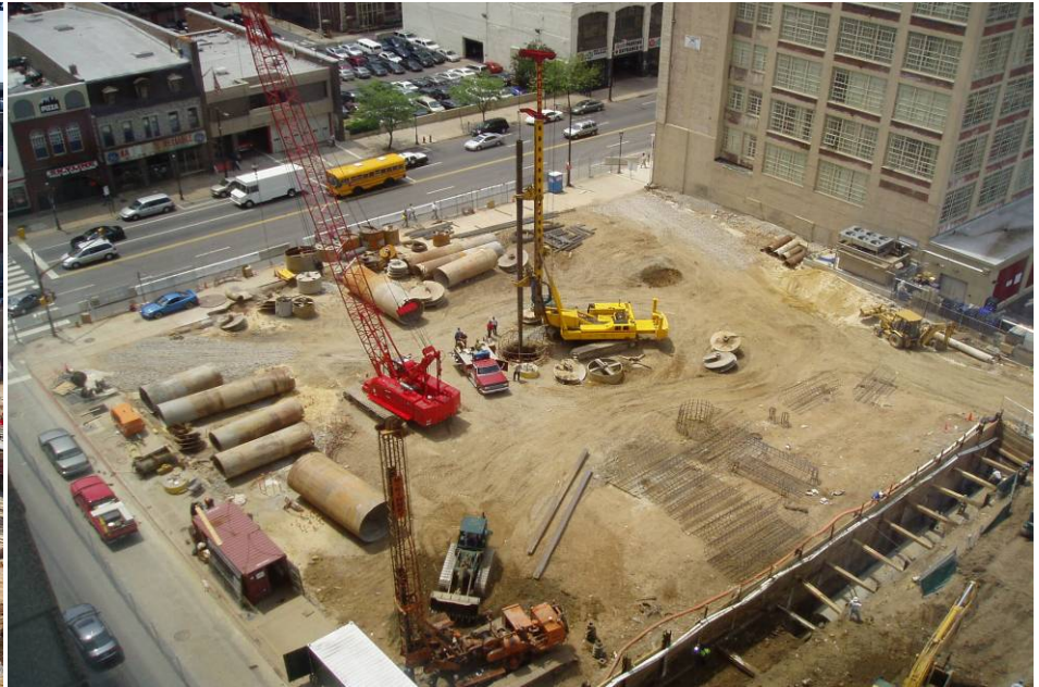
Case/McKinney Joint Venture 42 storey Condominium Tower, Philadelphia 8 feet diameter caissons 20 feet deep rock sockets
