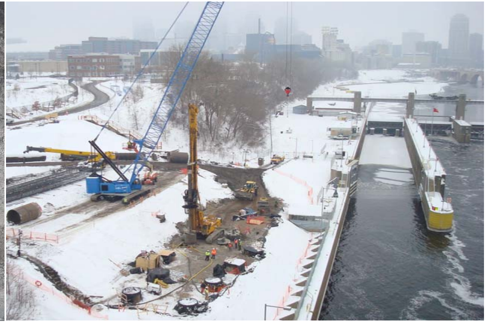
I35W, Minneapolis, Minnesota Bridge replacement Large diameter piles Joint venture Case & Anderson
