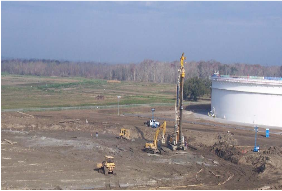
New oil storage tanks, South Louisiana Wet soil mixing Design & build. Repeat client Hayward Baker
