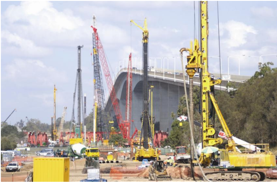
Gateway upgrade project, Brisbane, Queensland Several different products on site All four Australian companies contributing
