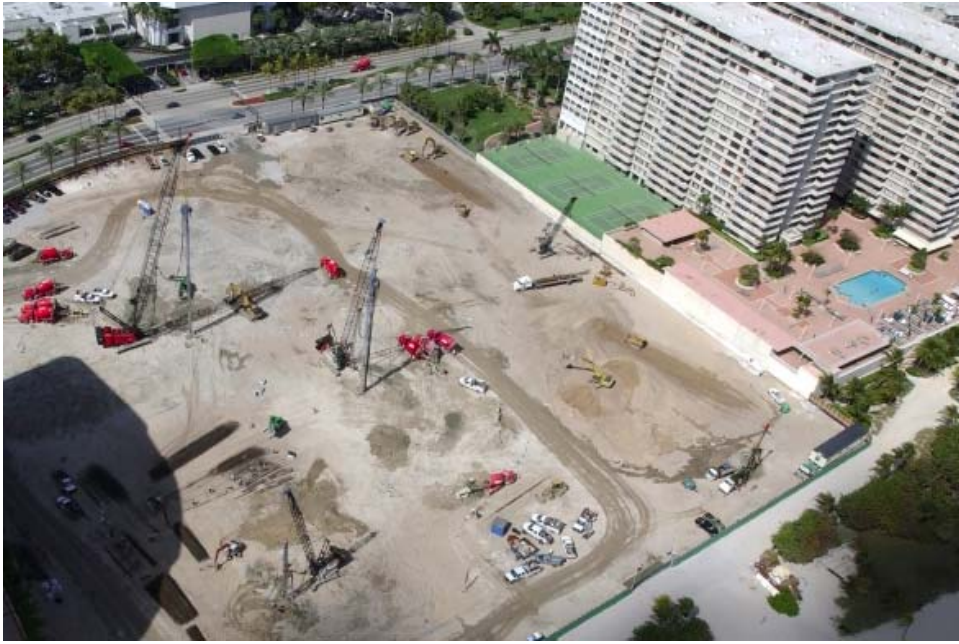
Foundations for a new hotel, Miami, Florida Continuous flight auger piling HJ Foundation
