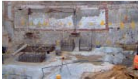
UK KGE uses "Soilcrete" jet grouting to underpin an eight-storey structure, allowing construction of a seven-metre deep basement at a London University building in Torrington Place, London.
