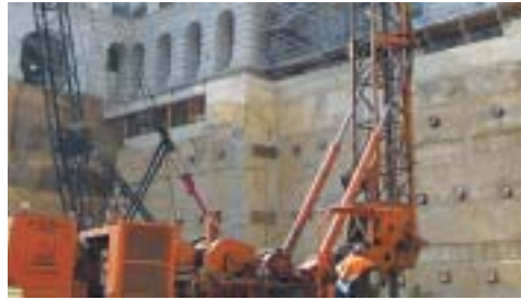
North America McKinney Drilling constructs drilled piers for the Capitol Visitors' Center, Washington DC.
