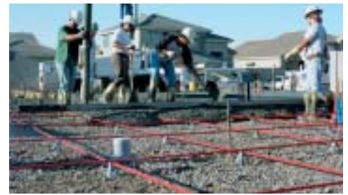
North America Concrete placement for a 190 mm post- tensioned foundation slab supplied by Suncoast for a single family residence in Phoenix, Arizona.
