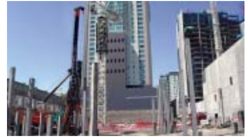
Australia Franki installs pre-cast piles for the 37-storey Melbourne & City Towers residential apartments in the Southbank area of Melbourne.
