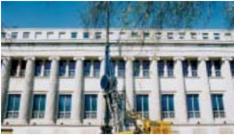
North America Case Foundation installs a reinforced concrete diaphragm wall and internal bracing system to allow construction of an underground storage facility at the Field Museum in Chicago.
