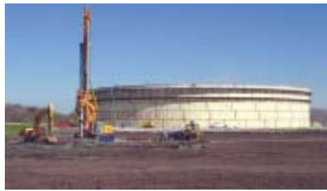
North America Hayward Baker uses 8-foot diameter soil mix columns to support 310-foot diameter oil storage tanks in marshlands in southern Louisiana.
