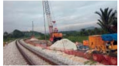
Far East Keller uses its "Vibro Replacement" technique to stabilise the foundations for the new high speed electrified railway line between Rawang and Ipoh in Malaysia.
