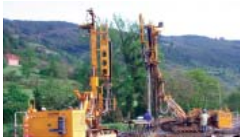
Europe Keller-Terra uses micropiles and horizontal drains to stabilise the slopes of the new Cantabrico Highway between Lieres and Villaviciosa in the province of Asturias, Spain.
