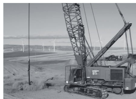
Above Dynamic compaction works for the Biglow Canyon Wind Farm in Oregon, US.
