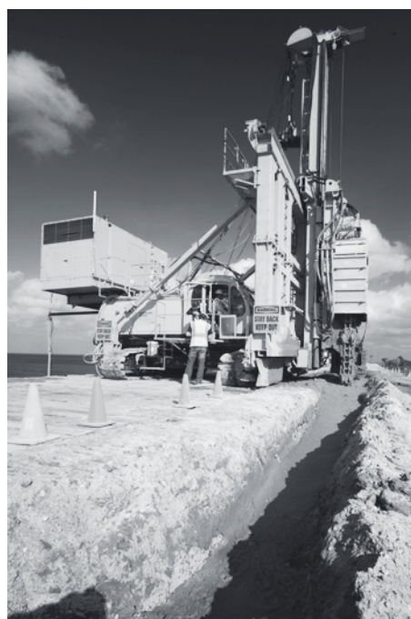
Below Creating a cut off wall within the levee around Lake Okeechobee in Florida, US.
